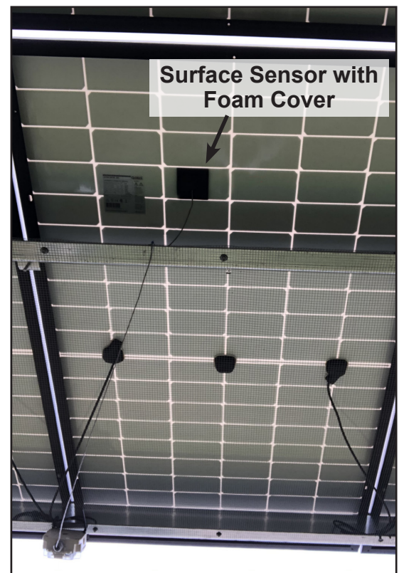
Fig. 3: Surface sensor installed on solar array.
